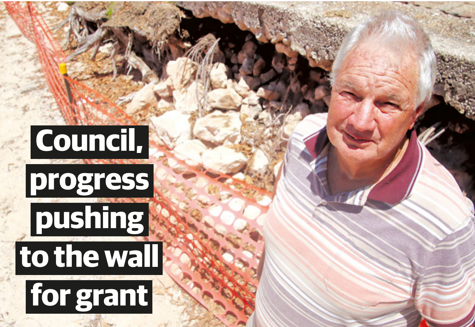
BREAKING DOWN... Stansbury Progress Association's Don McPhee is pleased Yorke Peninsula Council will pursue a grant to reconstruct the town's seawall, pictured behind him.
